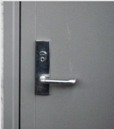
SECURITY FEATURE: LOCK TONGUE IS PROTECTED BY LEAF FRAME OVERLAPPING THE DOOR FACING
